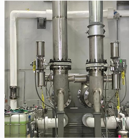
DOME heat rejection piping
