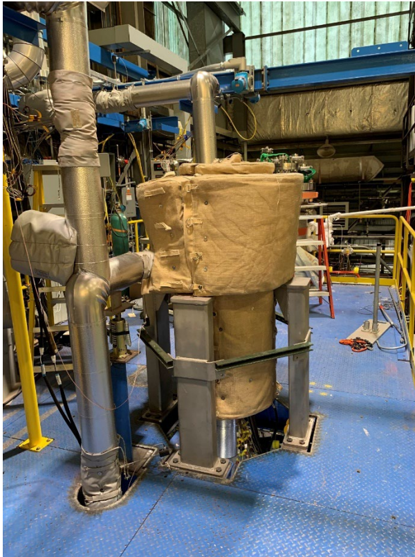
Figure 16: Test Vessel 6 - Installed
