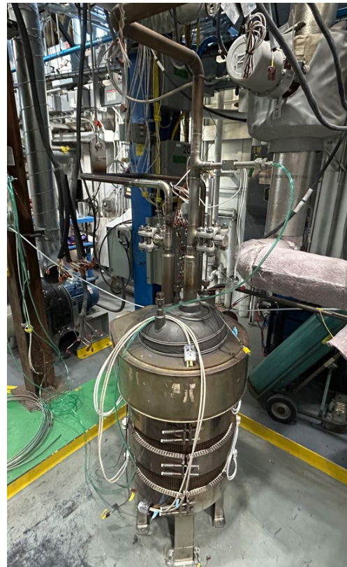
Figure 17: New Cold Trap Installed
