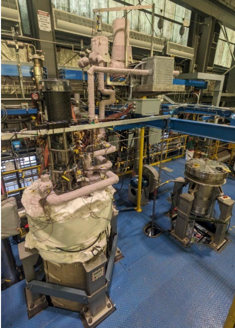
Figure 20 THETA fully installed in Test Vessel 4 (notice Test Vessel 6 to the right of THETA).
