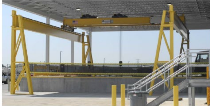
Figure 5-5. Free Standing Bridge Crane
