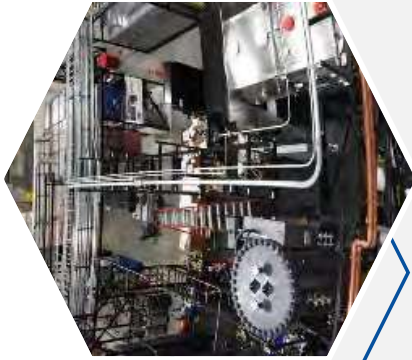
25 kWe High Temperature Electrolysis Stacks V&V
