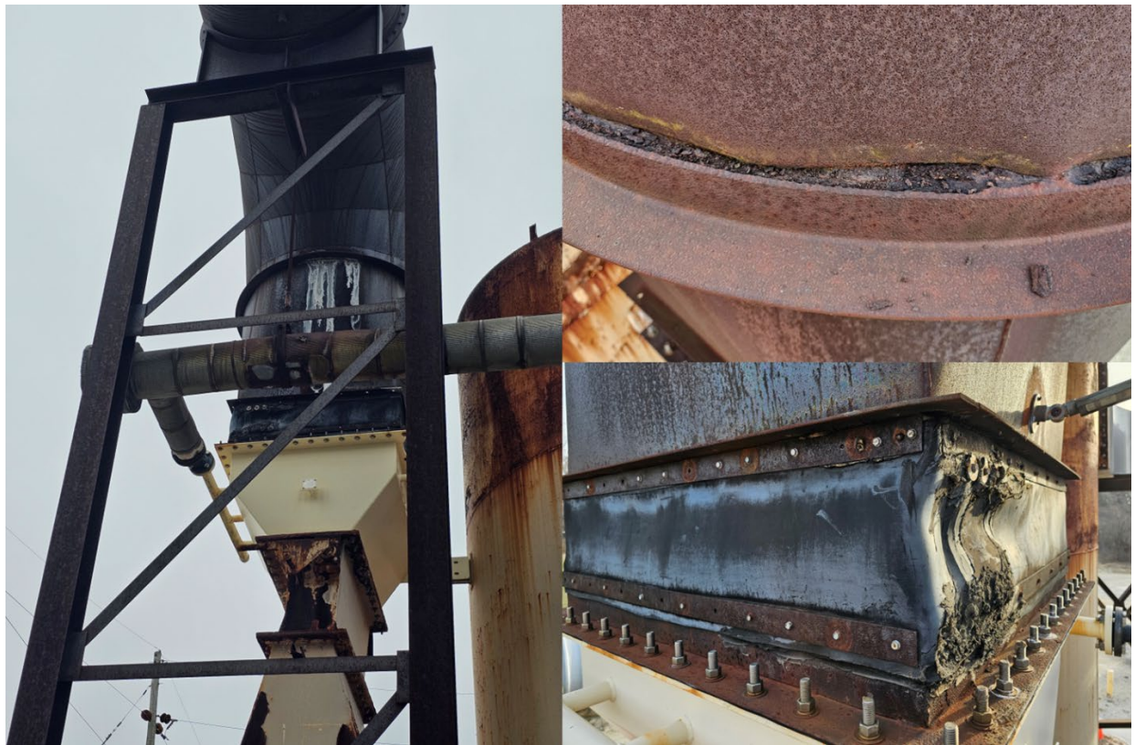
Figure 25 - Leakage from Duct Elbow (left), Broken welds on Elbow (top right), and Patched Expansion Joint (bottom right).
