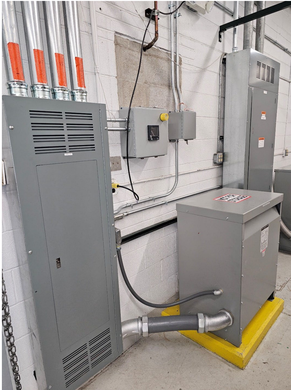
Figure 21. New Transformer and Panelboard for Experiment Support.
