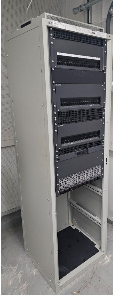
Figure 22. Centralized 24-Volt DC Power Supply
