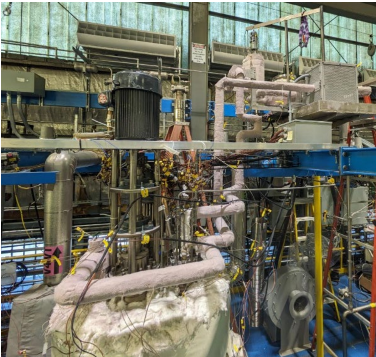
Figure 10. THETA with Secondary System Installed.
