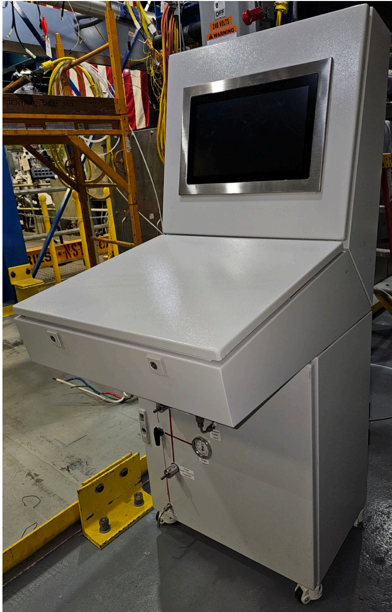
Figure 23 - Sodium Transfer Console (NaX).
