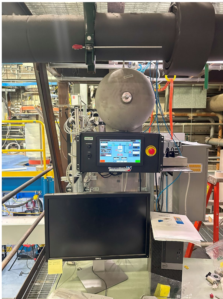
Figure 18. WVN Mixing Control Unit and Computer
