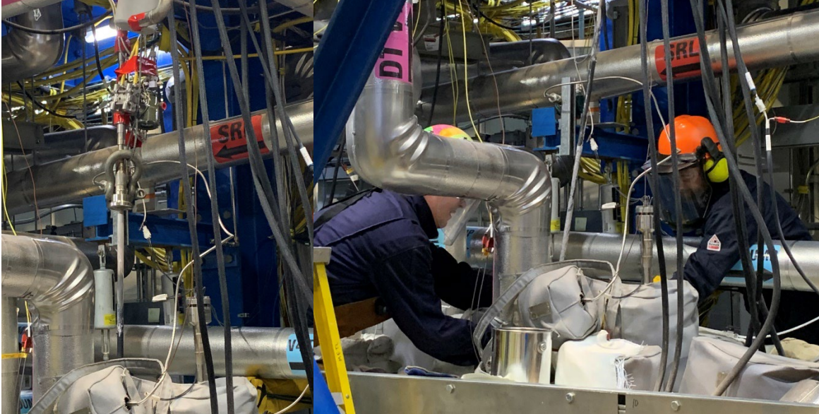
Figure 15. Differential Pressure Level Sensor Extraction (left) and METL Crew Members Installing Blind Grayloc Hub to Port (right).
