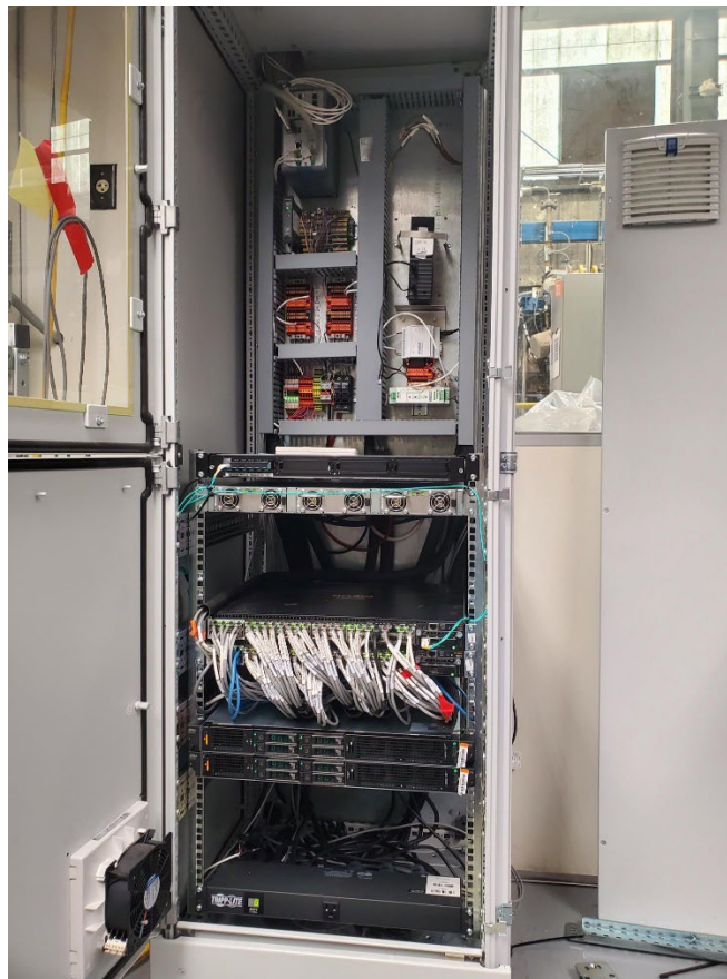
Figure 23. Servers Installed in Main Industrial Control Enclosure (2nd and 3rd Rack Mounted Devices form the Bottom).
