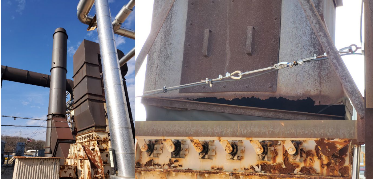
Figure 28. Original Corten Ducting (left) and Sheared Riser (right).
