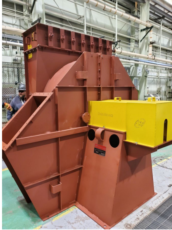
Figure 27. New 30,000 CFM Blower for B308 Alkali Metal Scrubber.
